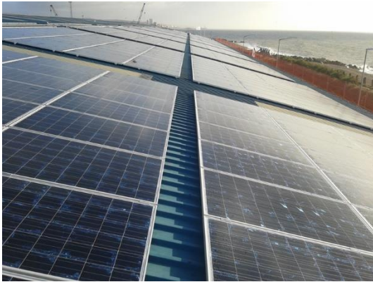
Solar panels on warehouse roofs
